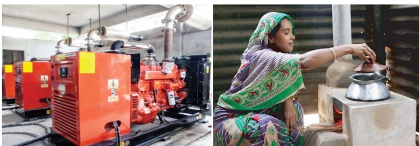
Left: Biogas based Electricity Generators at Gazipur (4 X 100 kW capacity).
