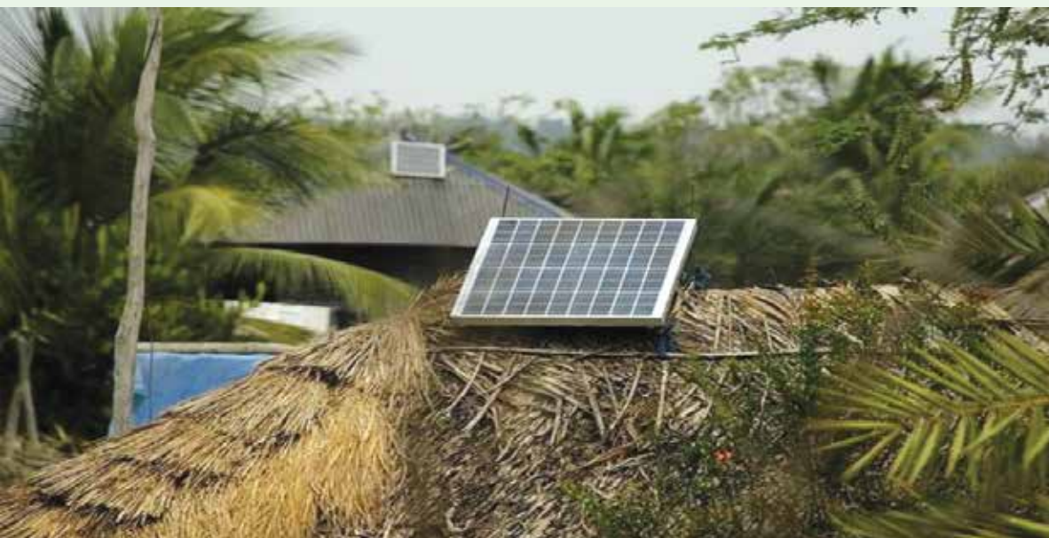
Solar Home Systemat Mirzaganj, Patuakhali
