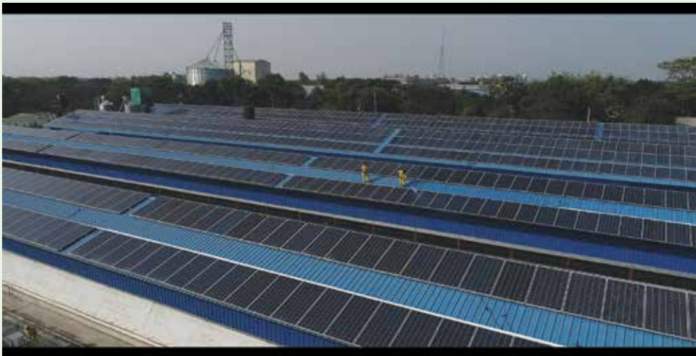
Rooftop Solar System
